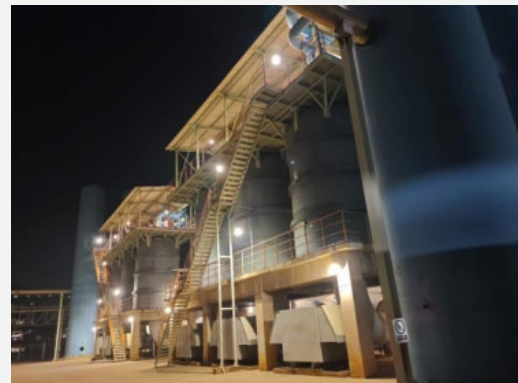
Oxygen Production System at the Lualaba Copper Smelter Plant
