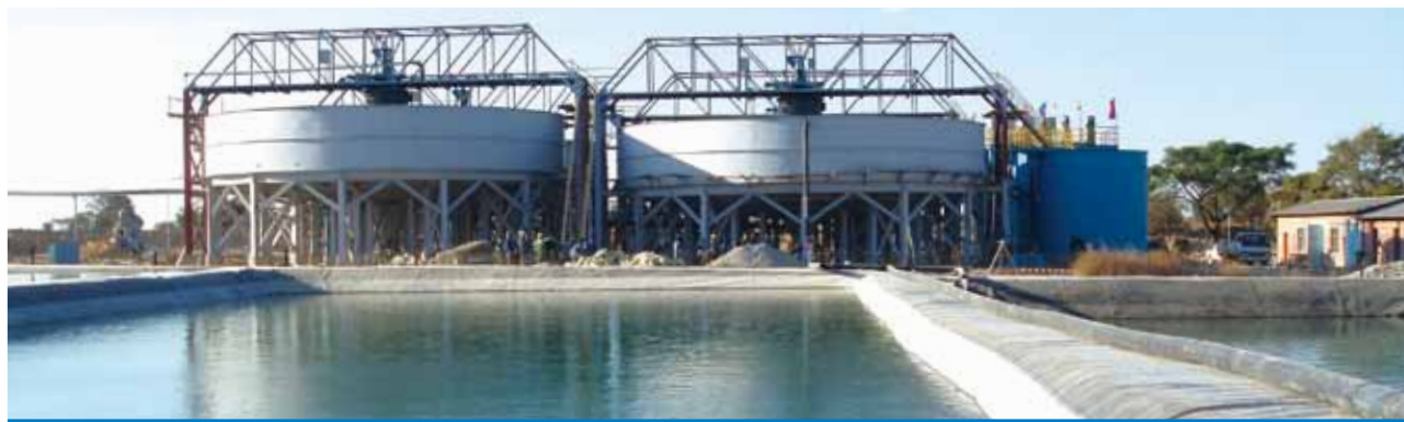
Settling pond for leaching
