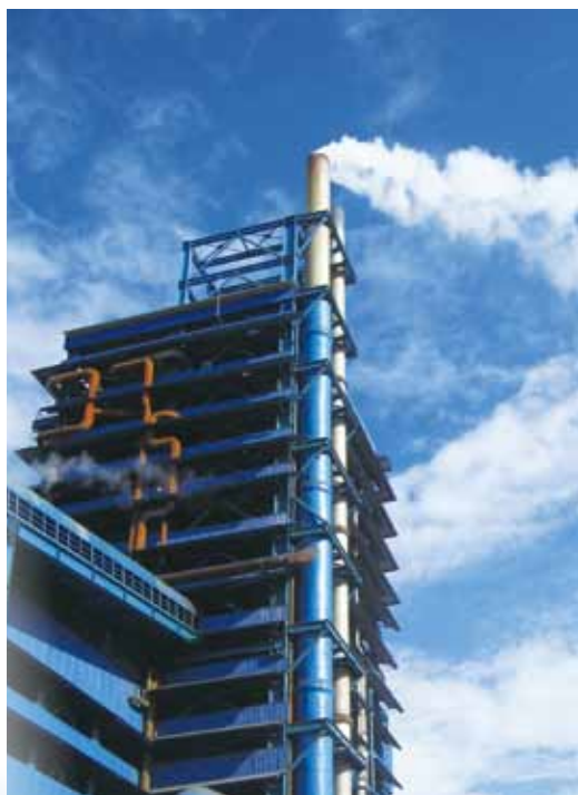
ISA furnace of copper smelting company
