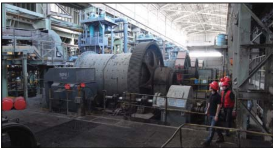
Figure 8-13: Ball Mills at Baluba Processing Plant
