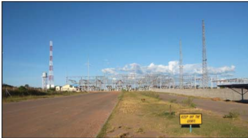
Figure 12-1: CCS 66/11kV Substation
