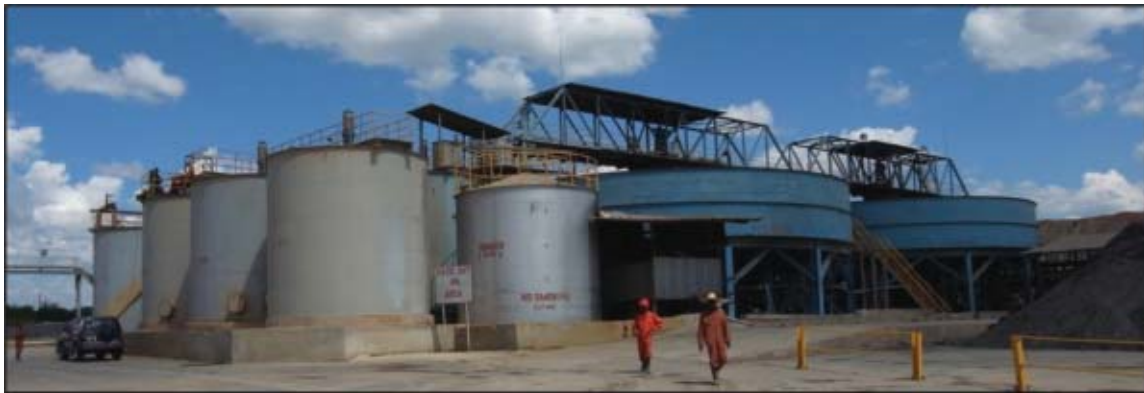
Figure 8-7: An Overview of Agitation Leach Plant
