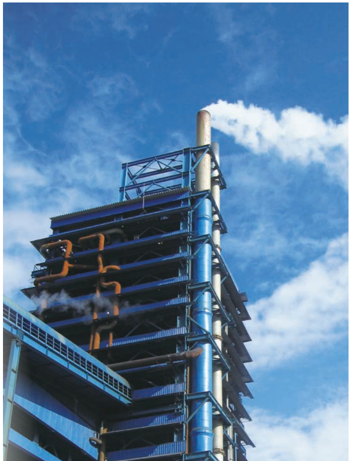
ISA furnace of copper smelting company
